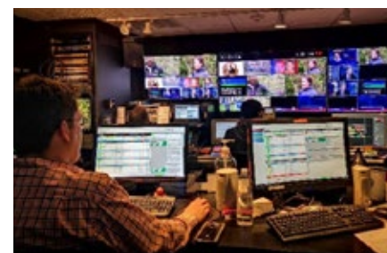
Control room at BRC TV
